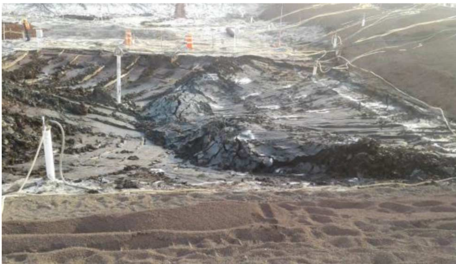
Figure 46. Semi planar failure mechanism of a trial excavation slope (Courtesy, W.I. Paniagua).
